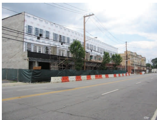
Prospect Avenue A and C buildings offering 14 mixed use units of which 7 are rental units and 7 are owner units.
